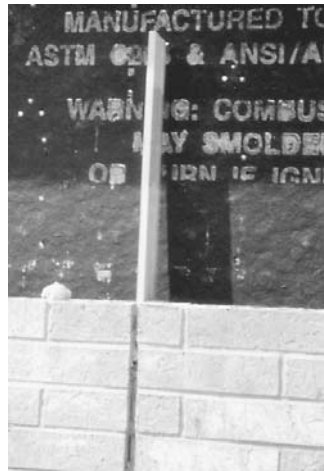
Figure 15-41 Remove boards or other non-compressible fillers used to keep mortar and debris out of expansion joints during construction.
